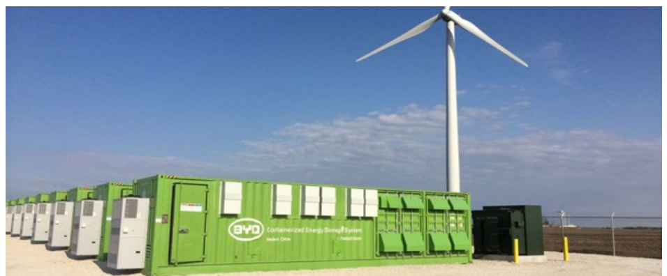
Grand Ridge battery storage facility | BYD
